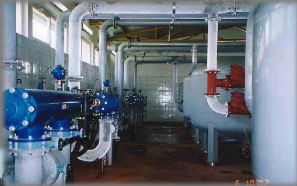
Bosna River Project—sand filters
